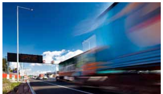
A view of the upgraded M1 Freeway technology in the heart of Melbourne's eastern suburbs.
